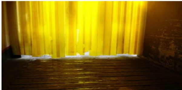
Damaged bottom of plastic strips doors allows pest
